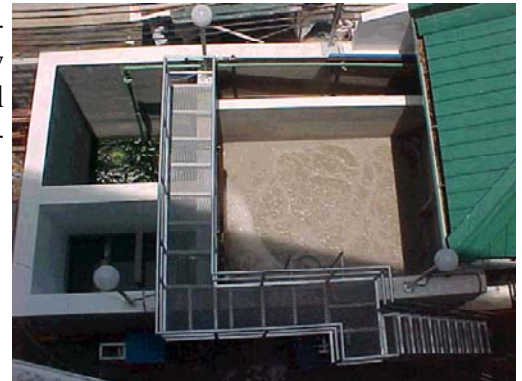
University Sewage Treatment Plant Capacity :85 m 3 /day.
