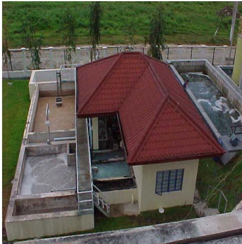
Bauer Dynamic Sequencing Batch Reactor(SBR) With Dissolved Air Flootation(DAF)
